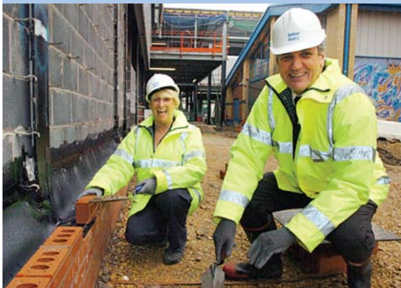
John Cuthbert, Managing Director, and Janet Bridges, Principal Designate of Castle View Enterprise Academy, laying one of the first bricks of the Academy's new building.
